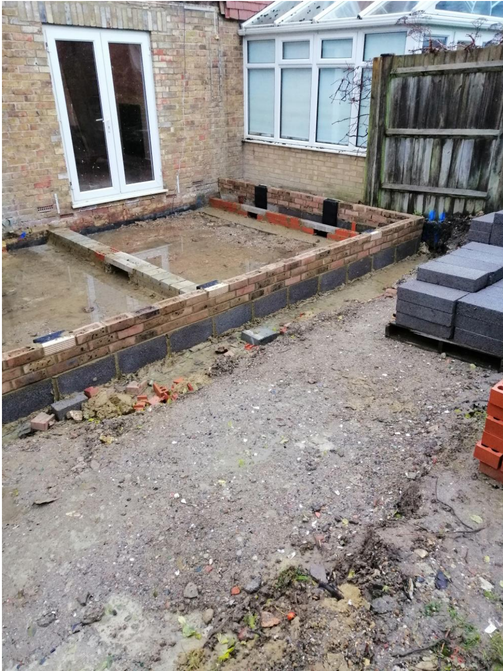
Why is water inside the extension but not on outside – is this surface water or water table
